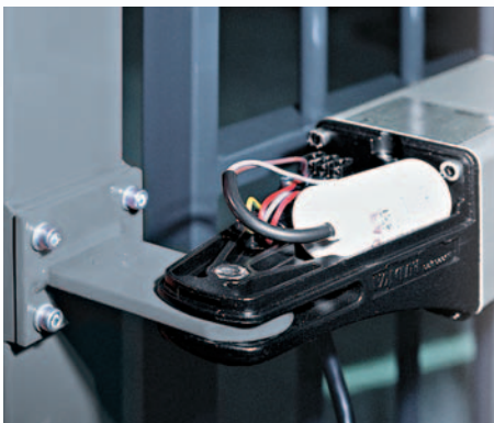
Detail of capacitor fixed into place
