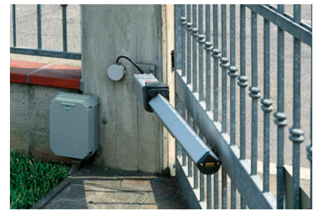
HINDI 880 installed on the gate
